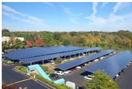
Photovoltaic installation in the company parking lot (United States)
