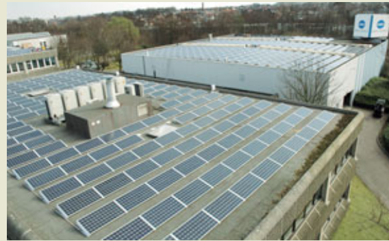
Solar panels installed on the roof of the company building
