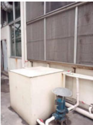
Window installed with evaporative air conditioning equipment and a recycled water tank
