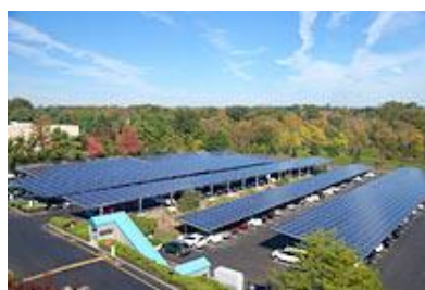
Photovoltaic installation in the company parking lot (U.S.)
