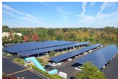
Photovoltaic installation in the company parking lot (The U.S.)
